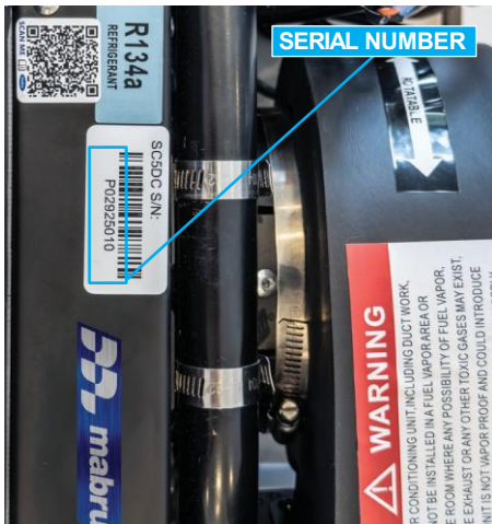
SN location on evaporator
